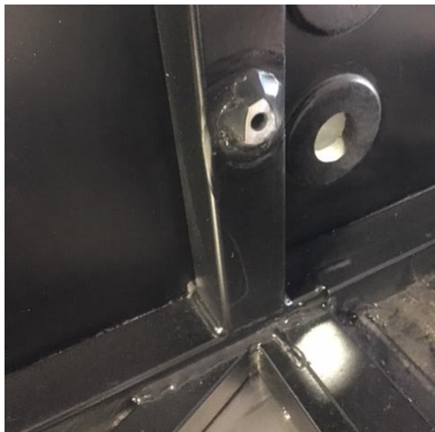
Figure 6 – Battery Ground Boss Location
